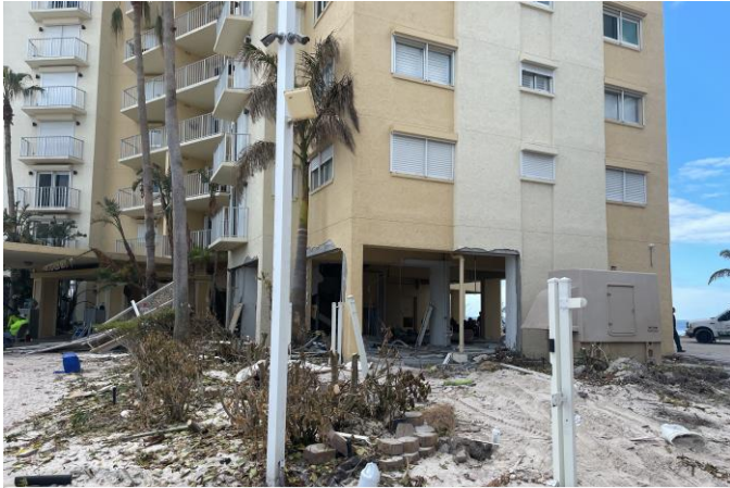
Surge damage to coastal properties in Vanderbilt Beach, FL
